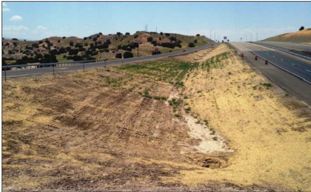
NM DOT revegetation demonstration trial plots two months after seeding on highway overpass construction project. From top to bottom: unfertilized control, concentrated compost, and NM DOT compost.
